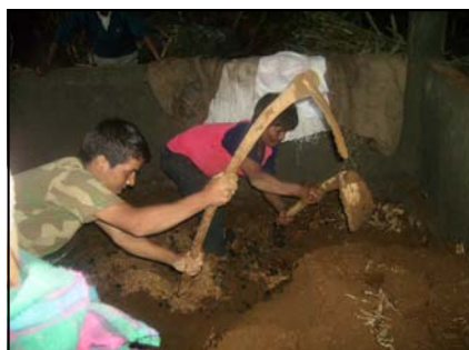
SHG members from Khrang village constructing a Bokashi pig shed. So far 12 SHGs have taken up Bokashi
